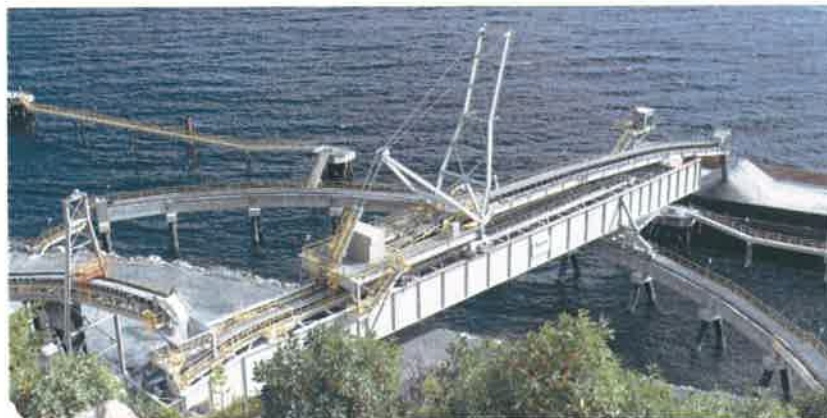
Figure 8: Texada Quarry (Lafarge) Shiploader
