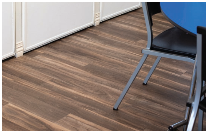
Before and after photos of flooring at the City of Pacific Senior Center. Updated flooring plays an important role in reducing falls and facilitating movement for seniors with mobility challenges.
