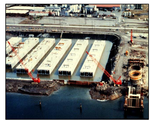
Flooding of the graving dock to launch Homer Hadley Bridge pontoons, Blair Waterway, 1981
