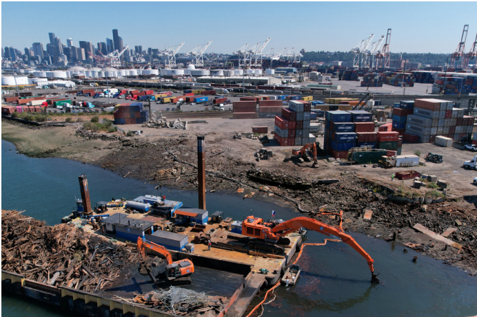
King County's Solid Waste Division is removing a derelict timber dock and its toxic, creosote-coated pilings from Harbor Island
