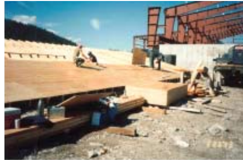
This is some of the prefab structure prior to lifting into place
