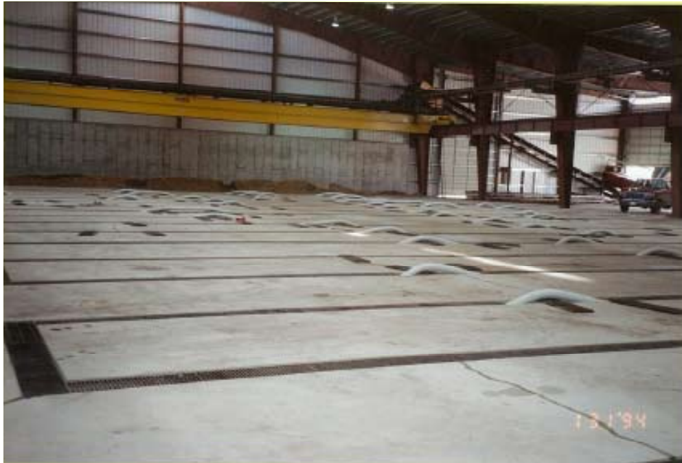
Aeration floor unit
