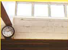
Leaky windows in library
