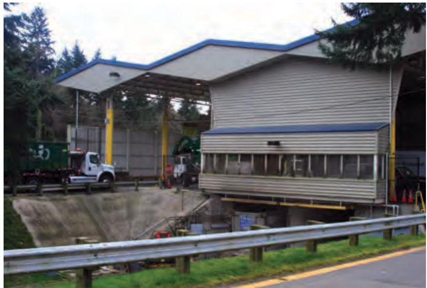
The roof at the Houghton Transfer Station was raised in 2012 to accommodate larger trucks
