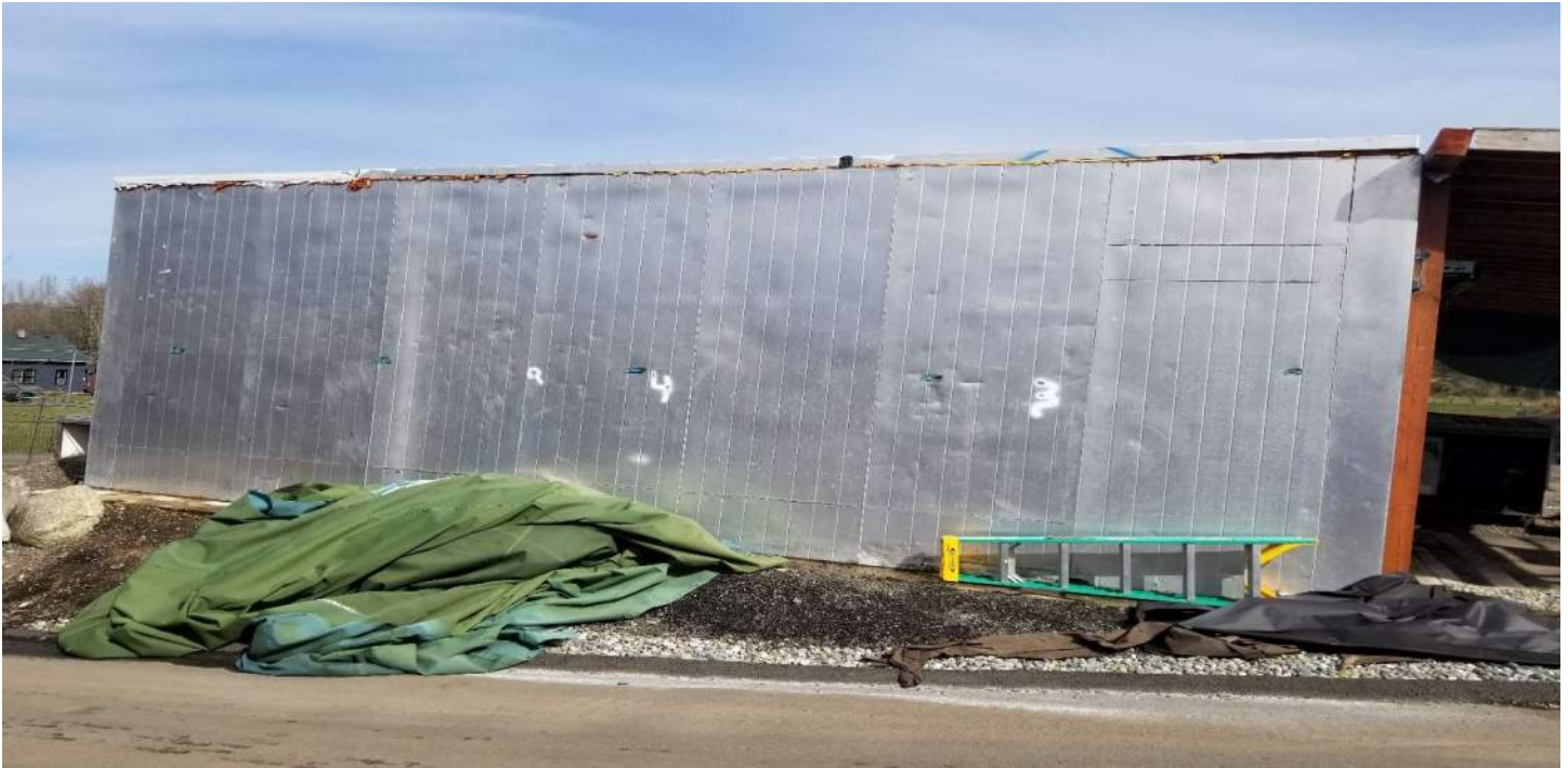
Above: freezer unit west side of freezer unit
