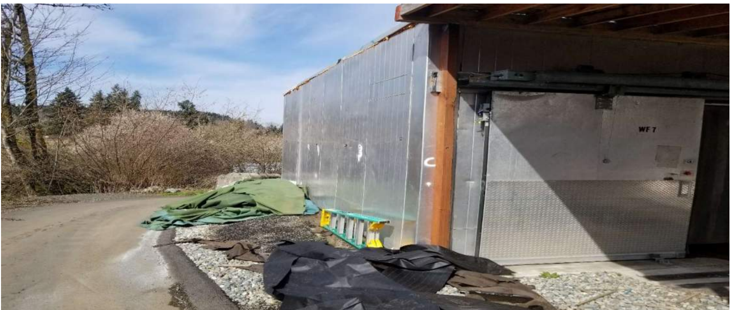
Below: Freezer unit west side of building
