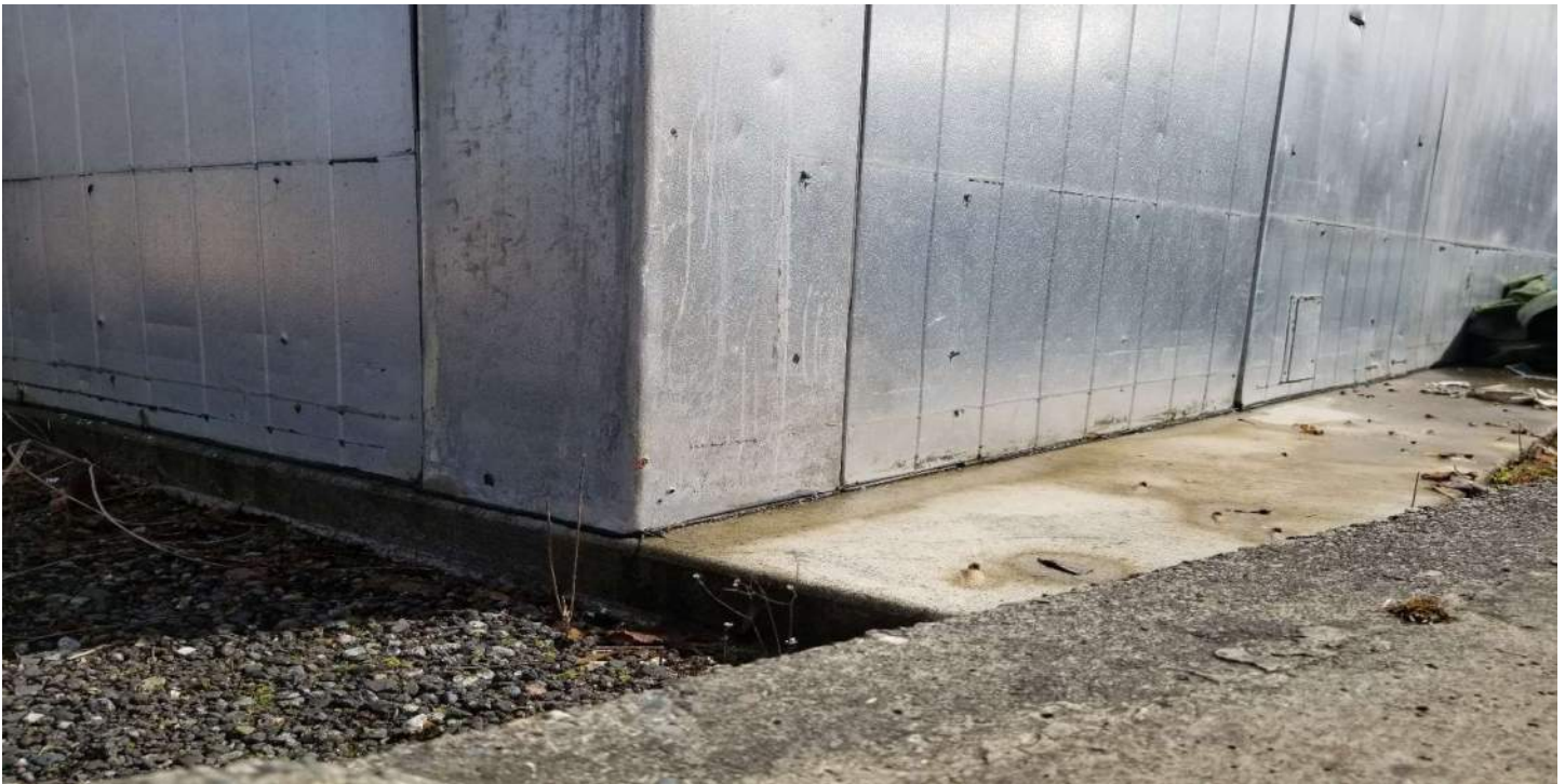
Below: Freezer unit 4" concrete pad below unit
