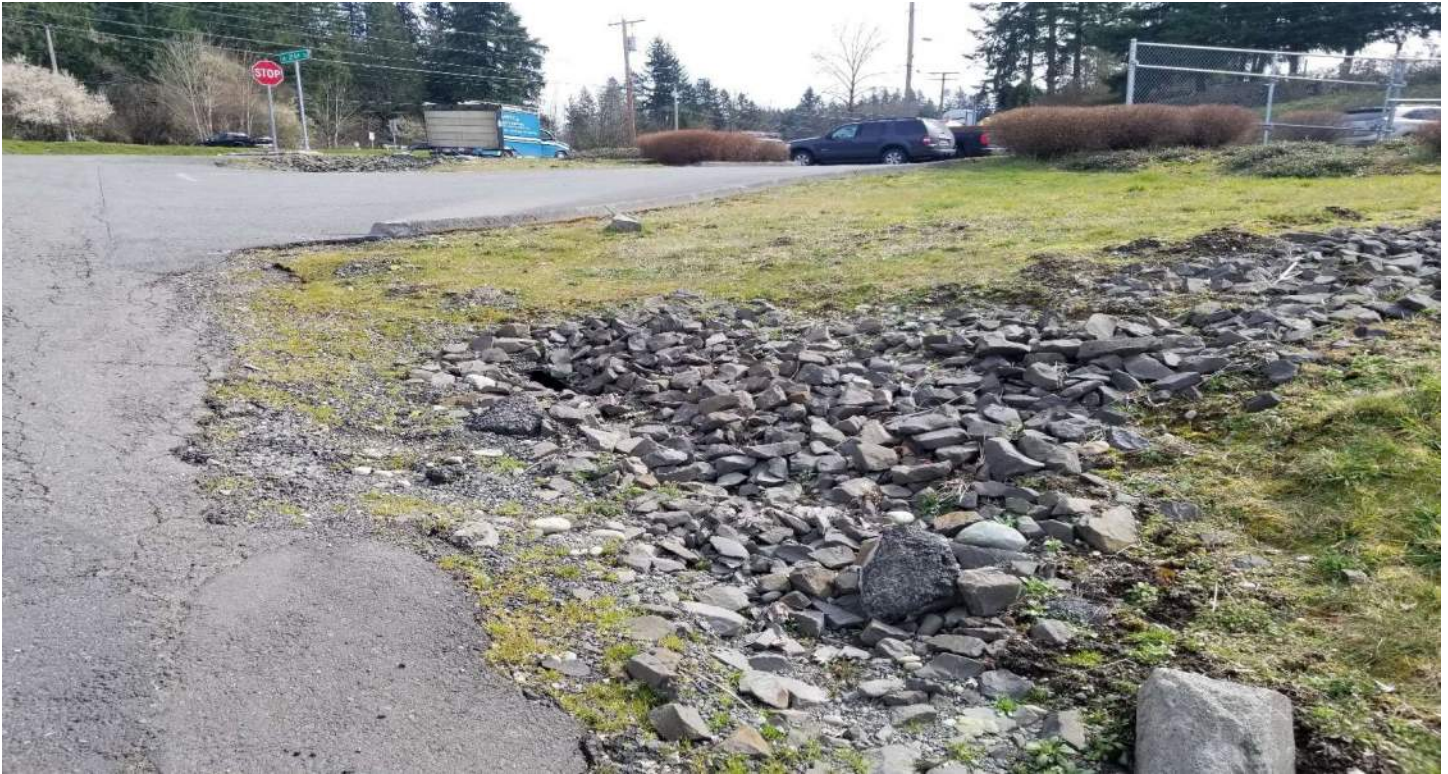
Above: Rip Rap Pad drainage from Renton Maple Valley Road and Parking Lot outfalls here
