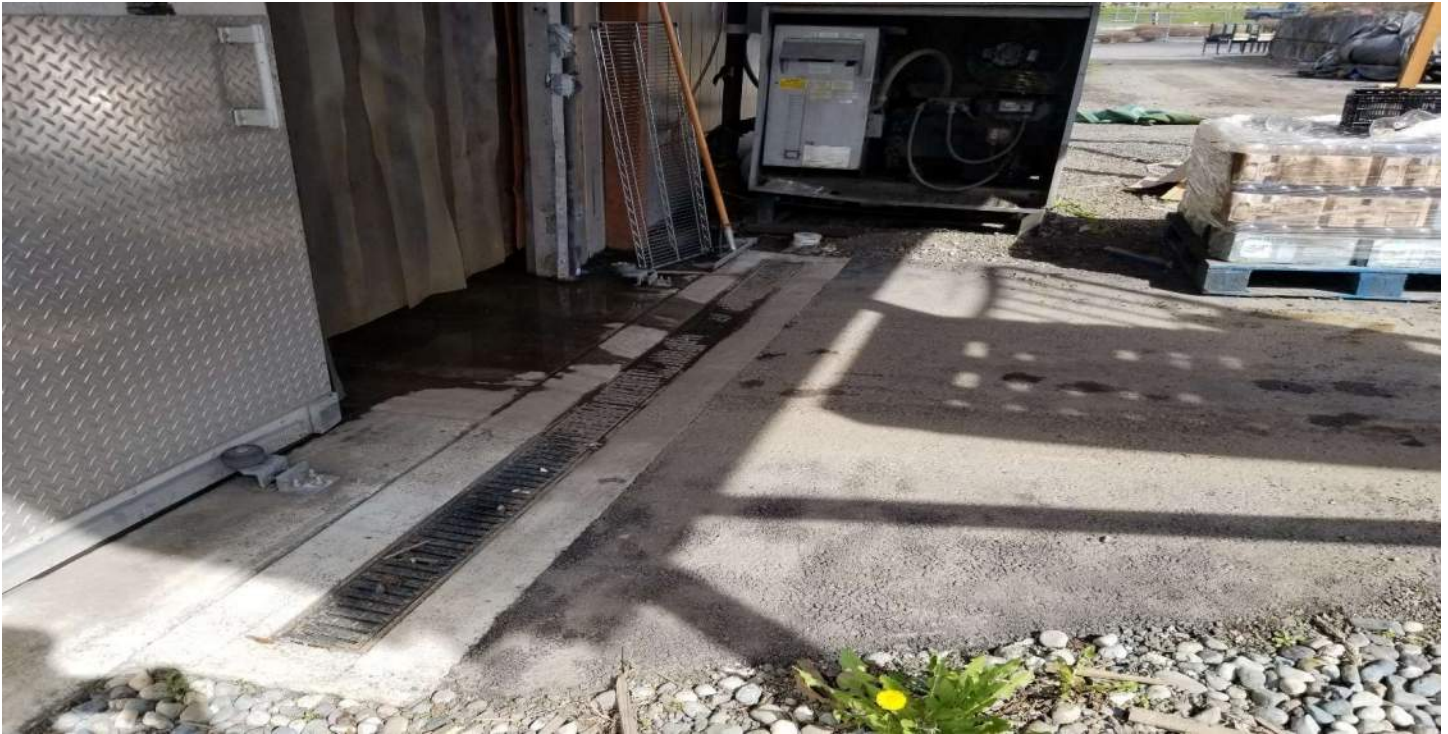
Above: Freezer unit French drain
