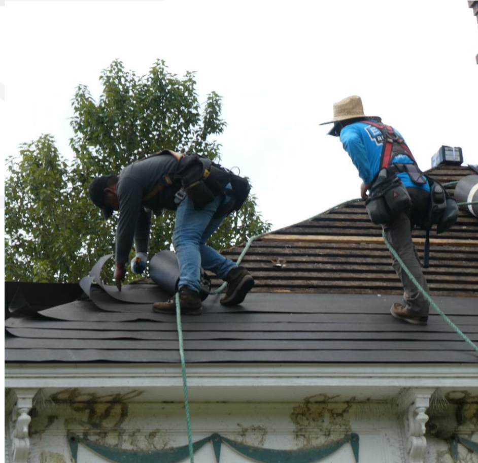
New overlapped felt paper was rolled out on top of the original skip jack boards (c) 2023, photo courtesy of Neely Mansion Association, Linda Van Nest
