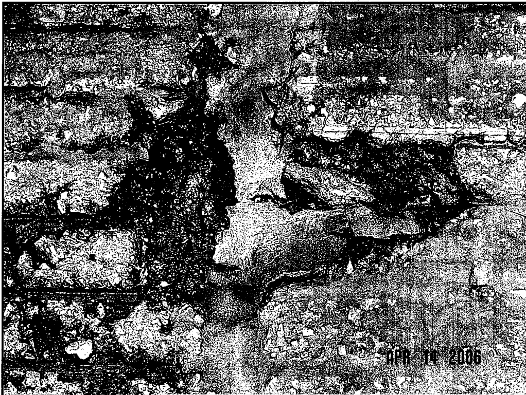
Figure 13: Pavement degradation generating FOD.
