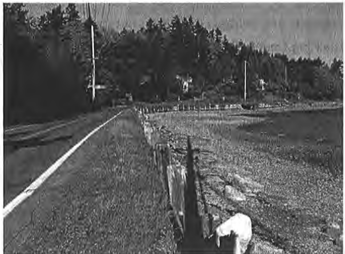
Dockton Road SW, located on Vashon Island in unincorporated King County, is protected by a 100-year old seawall that is vulnerable to storm surges and sea level rise.
