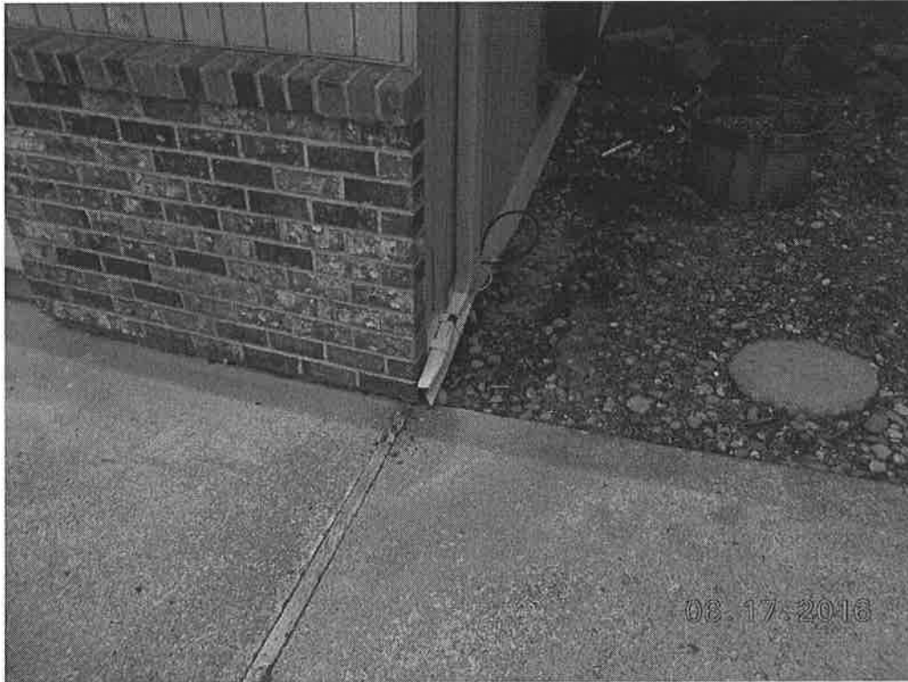
Photo 1: All downspouts discharge to the ground whether the surface is impervious like this downspout or pervious like the downspouts in Photo 2.
