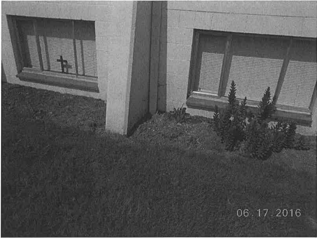
Photo 2: Downspouts on the southern building already go into the ground but it is not known what they are connected to.
