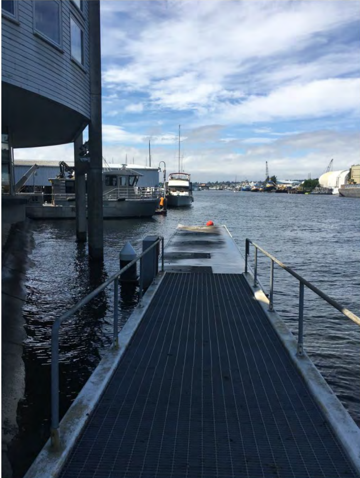
Figure 2 – King County bulkhead lease area. The SPU Dock (not subject to this lease) is shown in the foreground – the bulkhead lease area is in front of and to the left of the SPU dock in this photo (photo looking NW – taken 6-AUG-2021)
