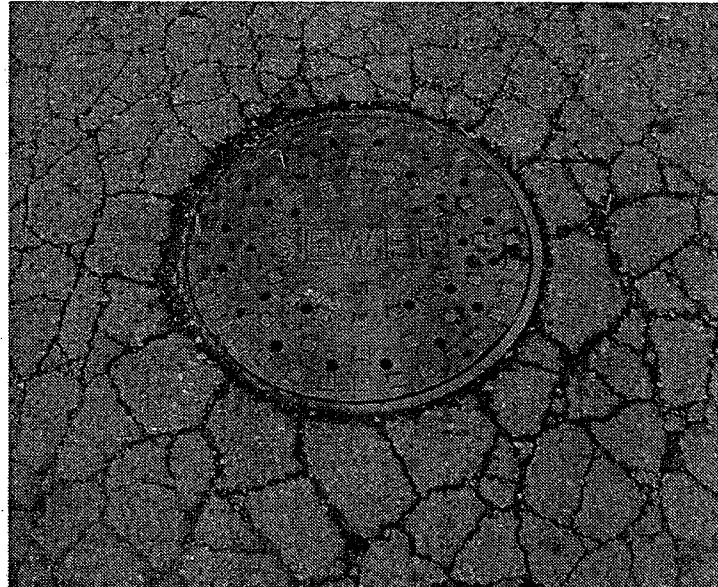
Manhole with indications of settlement in the pavement that likely subject the cover to inundation during rainfall. The large number of pick holes in the lid also allows free flow of surface water into the manhole.
