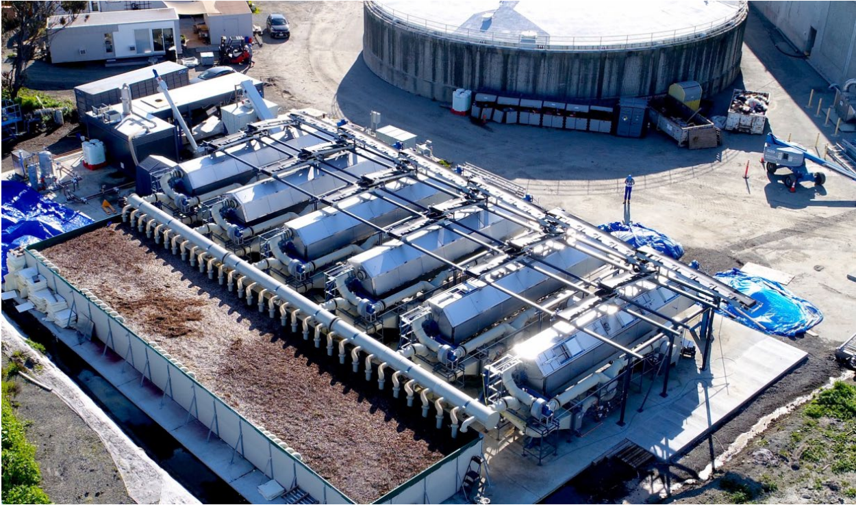
Figure 6. Silicon Valley Clean Water Authority biosolids drying and pyrolysis system
