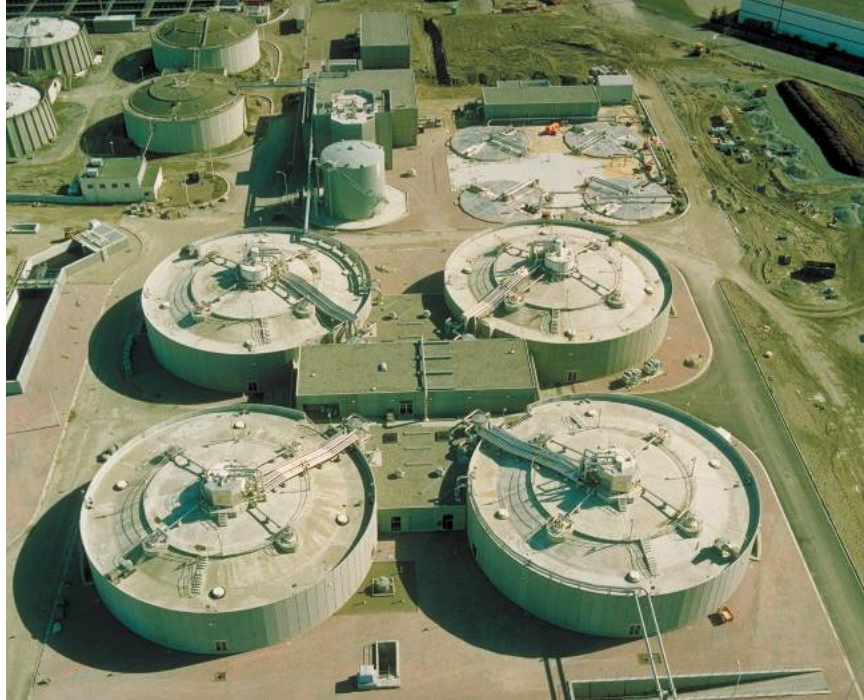
Figure 1. Thermophilic anaerobic digesters at Annacis Island WWTP
